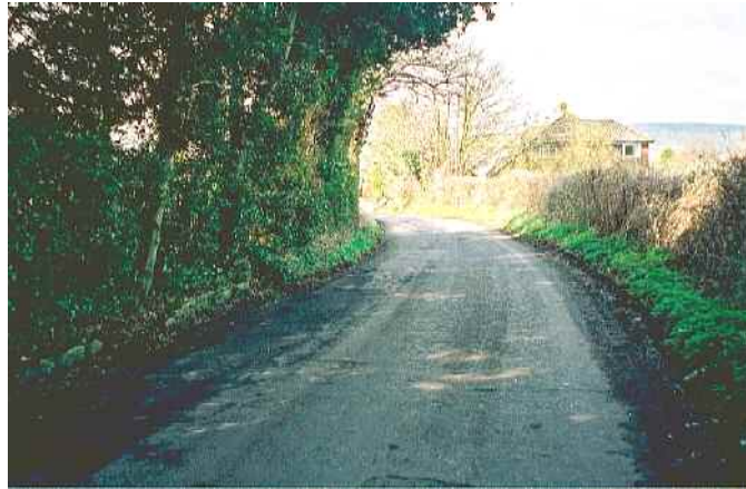
Figure 9: Surface deterioration following extended wet weather
