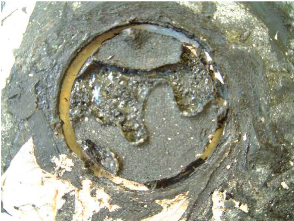
Figure 14. Failure of the sheet itself and of the bond of the sheet to the bonding bitumen
