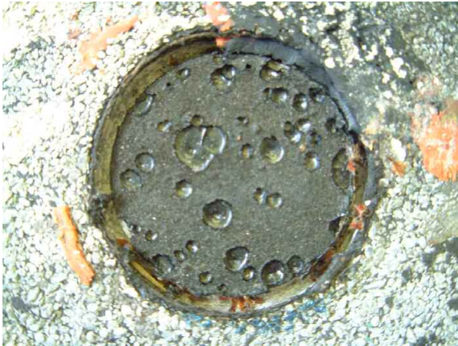
Figure 12. Typical failure surface at the interface between the sheet and the oxidised bitumen showing voids at the interface
