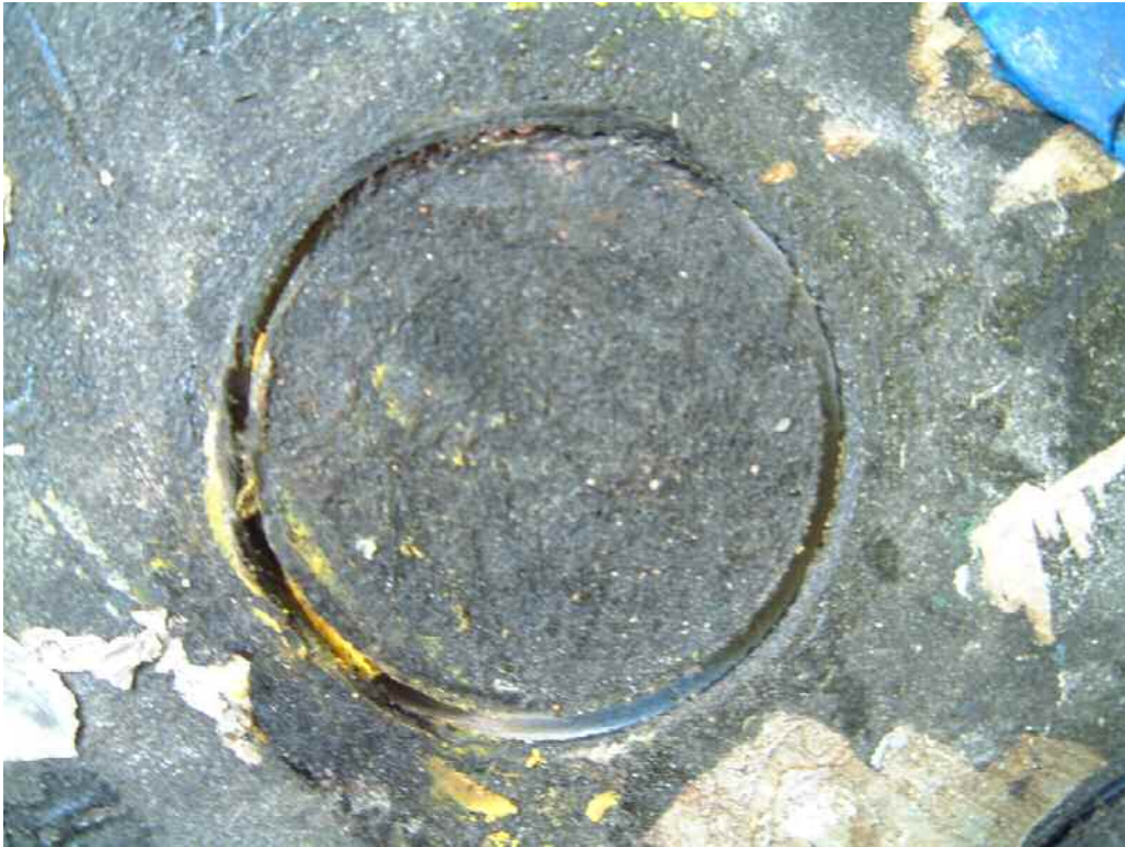
Figure 13. Typical failure at the surface of the sheet
