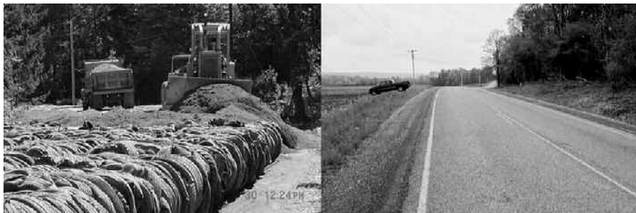
Figure 4. CR342 under construction (left) and in May 2004 after five years in service (right).
