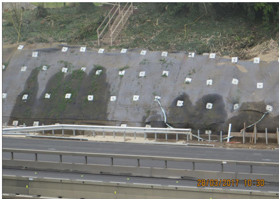
Figure 6: Seepages present on the cutting face at Cataractonium Cutting (image provided by National Highways)
