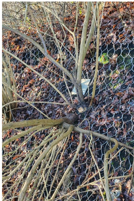
Figure 17: Vegetation growing through the mesh on the soil nail slope at M6 Junction 10 (image the authors)
