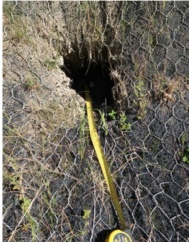
Figure 11: Mesh soil nail slope facing where slope movement forces have caused punching failure of the soil nail mesh facing. After failure the face plate is approximately 600mm behind the facing (image the authors)
