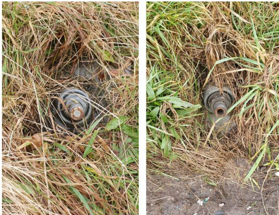
Figure 14: Soil nail heads on the A628 east of Manchester showing varying amounts of grout loss from within the nail head (image the authors)
