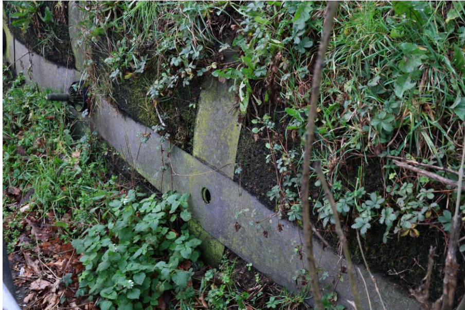
Figure 18: Missing soil nail from a slope adjacent to an emergency layby along the eastbound carriageway of the A42 (image the authors).
