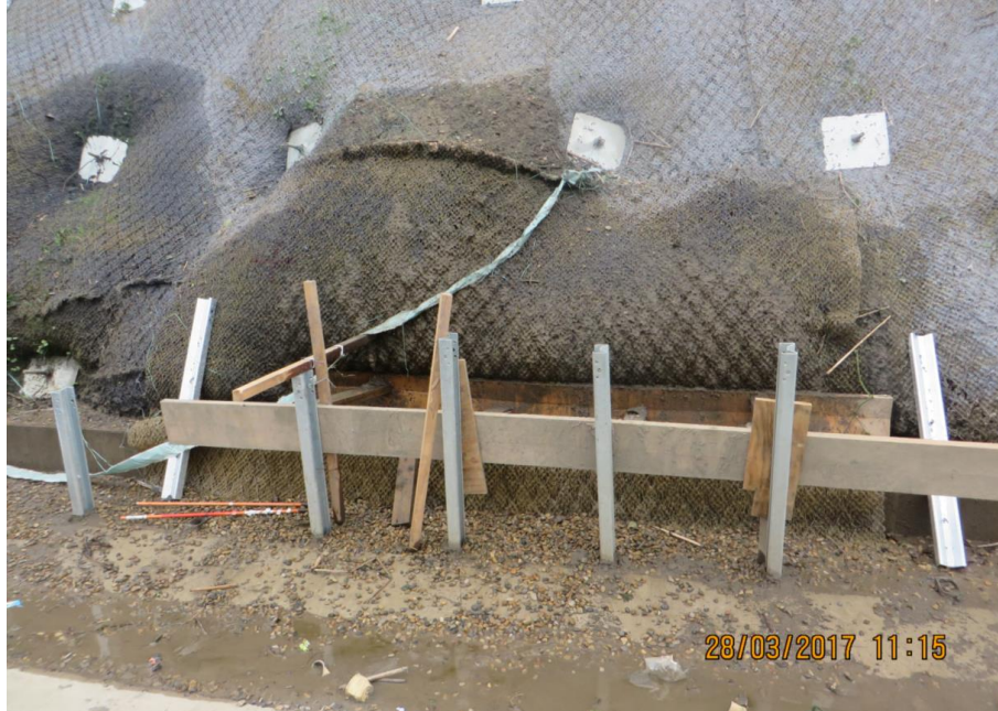
Figure 9: Slumping of the soil nail slope (SNS2) causing deformation of the facing at Cataractonium Cutting (image provided by National Highways)
