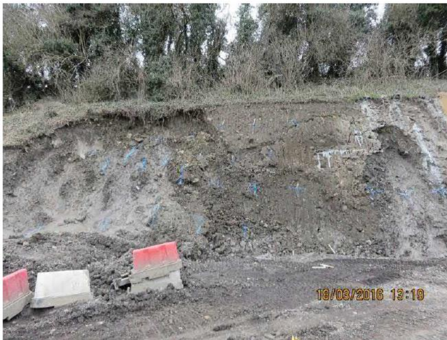
Figure 2: Failure of a full height slope excavation prior to installation of the soil nails, A1 Dishforth to Barton Improvement (from Carillion/Morgan Sindall JV, 2018)
