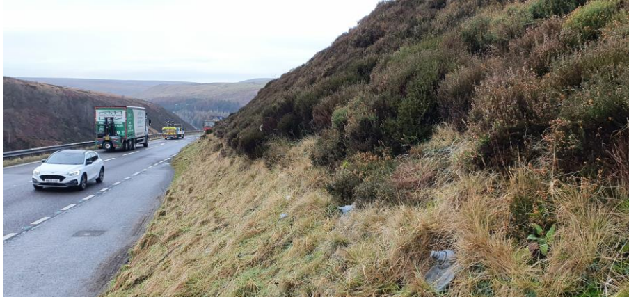
Figure 13: Soil nails installed in cutting adjacent to layby on the A628 to the East of Manchester (image the authors)
