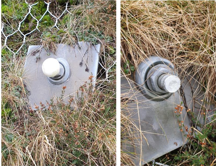
Figure 15: Soil nail heads on the A628 east of Manchester with rare caps present. The image on the right shows the condition of the nail head beneath a cap indicating no corrosion or grout loss (image the authors)
