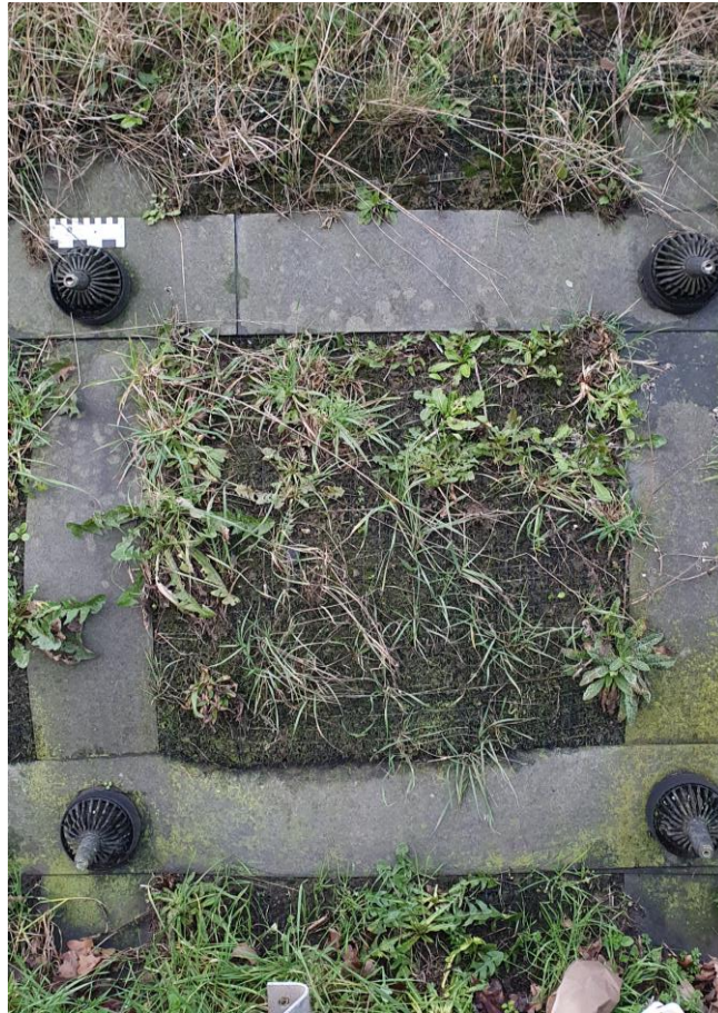
Figure 10: Facing of a soil nail slope comprising concrete cloth straps/planks with a small aperture black geogrid, A42 northeast of Ashby-de-la-Zouch (image the authors)
