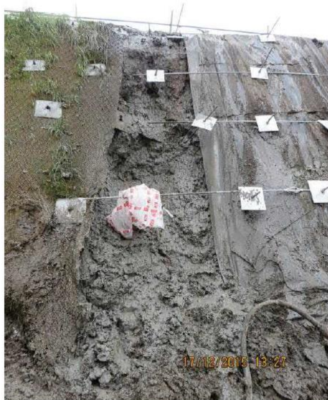
Figure 3: Failure of a slope which was left partially nailed and partially faced over an extended period, A1 Dishforth to Barton Improvement (from Carillion/Morgan Sindall JV, 2018)
