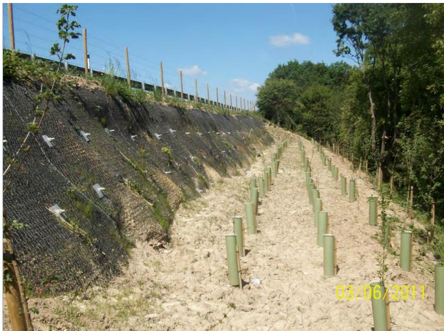
Figure 1: Failure of a soil nail slope after construction with bulging between the nails, A21 Lower Haysden (from Balfour Beatty Mott MacDonald, 2013)
