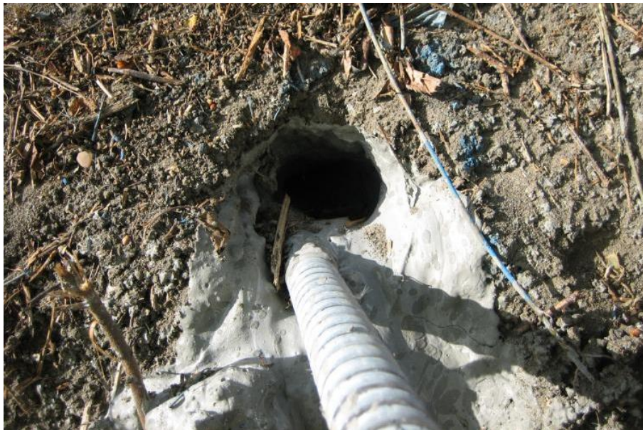
Figure 4: Self-drilled soil nail lying on the base of the borehole due to failure to use centralisers. This reduces the grout cover for corrosion protection and potentially reduces the bond strength (image the authors)
