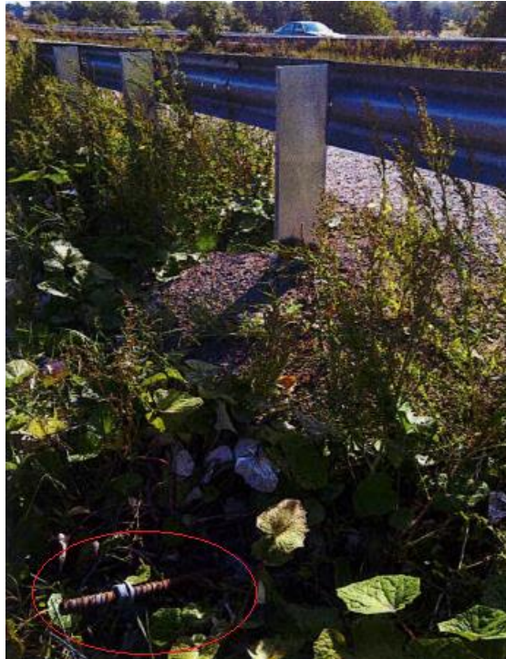
Figure 16: Soil nail protruding from the face directly below a safety barrier post which was installed at a later date, M23 Gatwick Spur (from Balfour Beatty Mott MacDonald, 2011)
