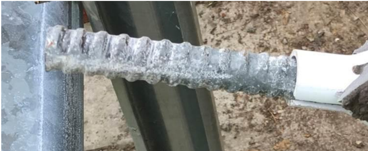
Figure 19: Presence of white substance on the soil nail tendon following pull out of the soil nail at the Cataractonium Cutting (image provided by AECOM).
