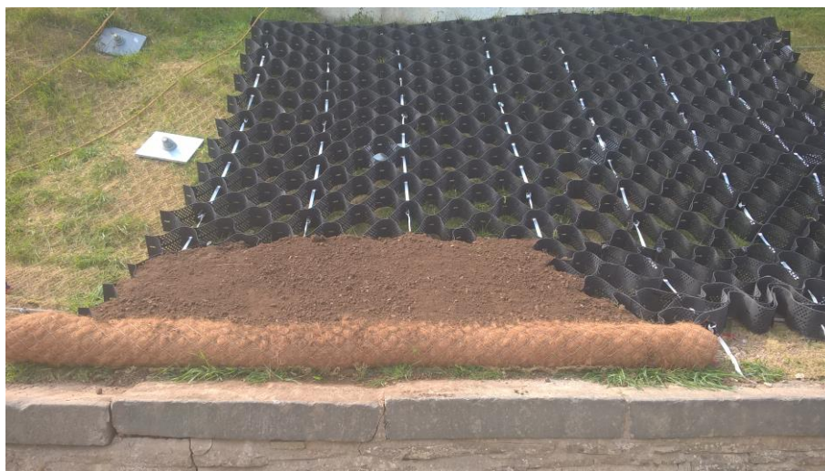
Figure 12: Geocell installed on a soil nailed slope and infilled with topsoil to prevent a trip and spike hazard in a publicly accessible area (image the authors)
