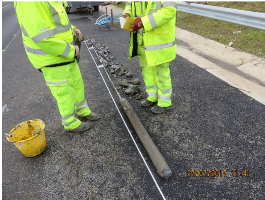
Figure 5: Extraction of soil nail as part of the forensic investigation. The nail was pulled out of the slope with a load greater than required by the acceptance tests (image provided to Coffey by AECOM in 2017)
