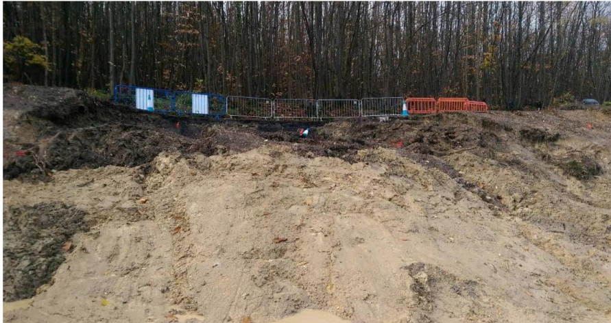
Figure 8: Failure of a partially soil nailed slope during construction, A21 Tonbridge to Penbury (from WSP, 2019)
