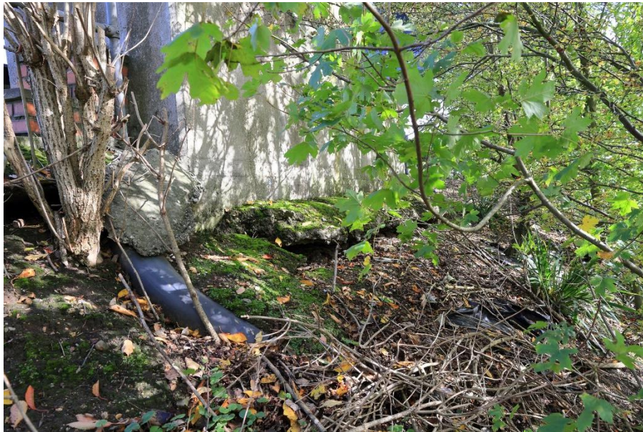
Figure 16: Slope above the 'Porcupine' modular concrete Block Walls (Figure 2) showing settlement beneath the foundation for a variable message sign and significant long-term twisting of tree trunks indicating a wider instability issue (A1307 (formerly A14), above SGM 6082 (Gabion wall), October 2020).
