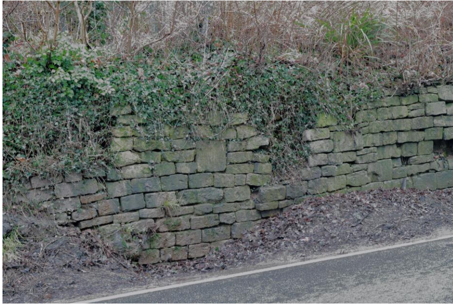
Figure 19: Dry stone wall showing significant signs of instability (A36, SGM 9077, January 2021).
