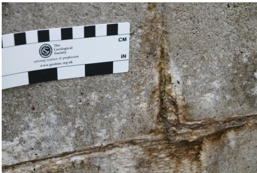
Figure 12: Concrete block wall showing what appears to be efflorescence in the blocks and particularly in the mortar (A38, SGM 10857, January 2021)
