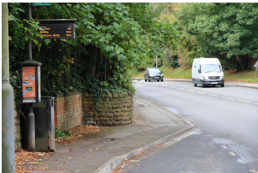
Figure 13: Mortared stone block wall up to 1.7m high showing signs of leaning, block and mortar loss. Brick infills seem to coincide with former driveways; where the block wall is now retaining this may not have been the case originally (A52, SGM 9676, October 2020)
