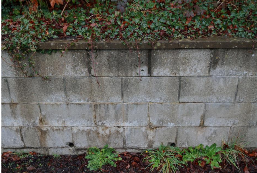
Figure 11: Weepholes (50mm internal diameter) in a 57m long, 1m high concrete block wall. The weepholes were observed to be functional, and what appears to be efflorescence was observed in the blocks and mortar (A38, SGM 10857, January 2021)
