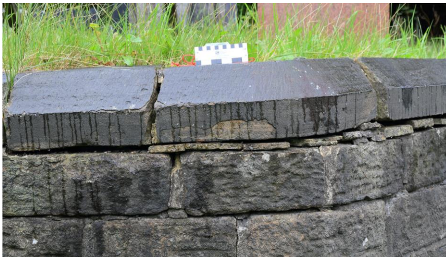
Figure 2: Deterioration and mortar loss of the top course of a stone block mortared retaining wall (A628, SGM 8885 [unique SGM code from Atkins/Jacobs, 2020], October 2020)
