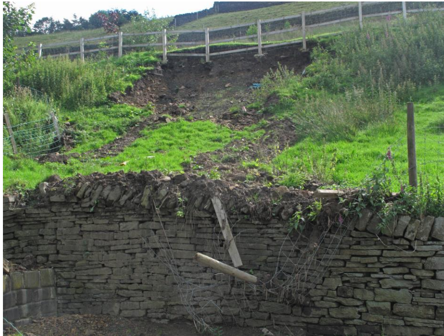
Figure 14: Dry stone retaining wall approximately 1.2m height that has been affected by the failure of the slope above (off network, West Yorkshire, August 2012)
