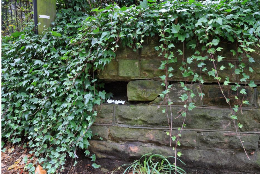
Figure 3: Deterioration of the lower courses of a stone block mortared wall seems most likely due to salt spray. The deterioration of this wall at this location is through the full height with the loss of block(s) in the central area (A52, SGM 9676, October 2020)
