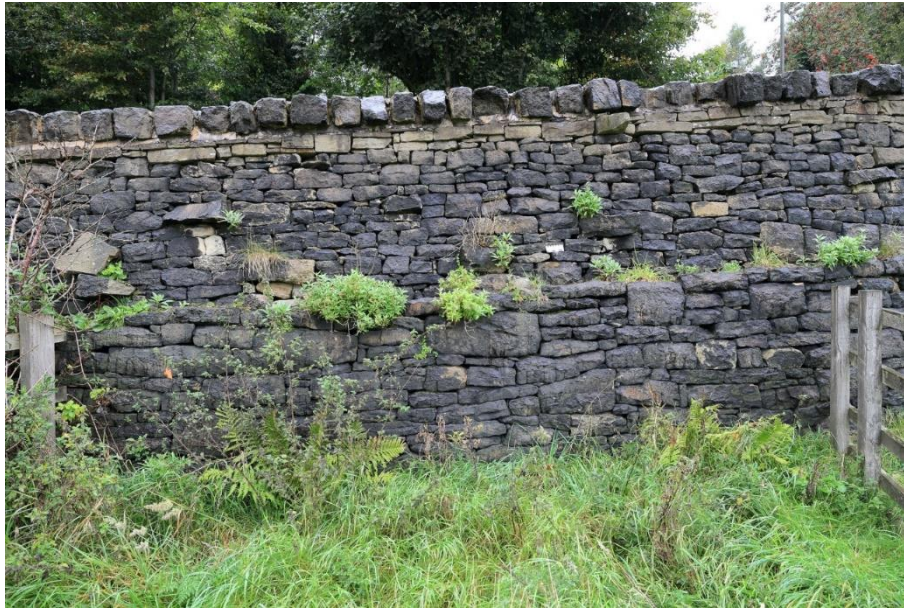
Figure 15: Dry stone wall approximately 2.5m high including 0.5m free-standing (A628, SGM 8923, October 2020)
