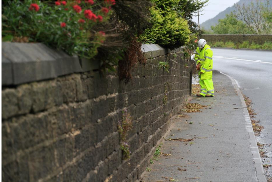
Figure 7: Leaning stone block mortared wall of approximate height 1.65m. Signs are also evident of bulging and deterioration (including mortar loss) of the top course. Note the change in angle of the masonry courses, the angle between the courses and the coping stones and the vertical alignment of the highway (A628, SGM 8885, October 2020)
