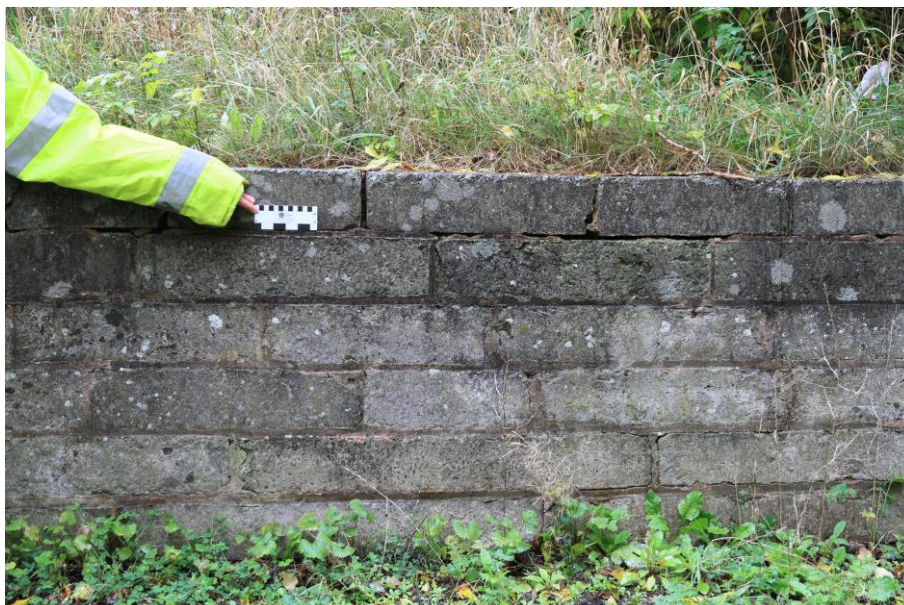
Figure 9: Mortared concrete block retaining wall, approximately 0.9m high along base of embankment showing signs of bulging, leaning and deterioration of top course (A52, SGM 7825, October 2020)
