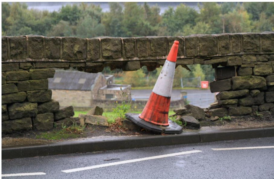
Figure 4: Upper free-standing part of a dry stone retaining wall (mortared coping) showing the effects of vehicle impact. The wall below the carriageway retains a height of between 2m and 3m below the road. (A628, east of SGM 8885, October 2020)
