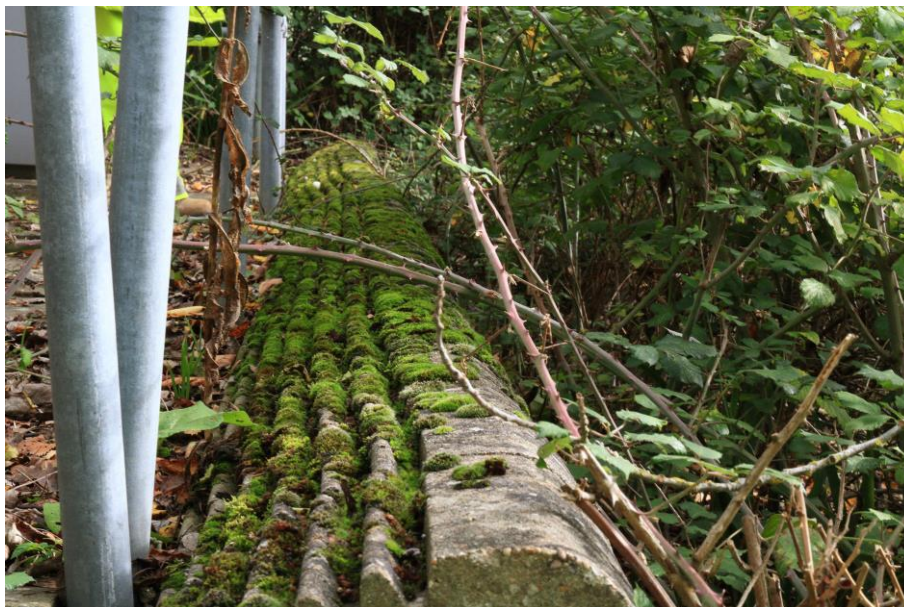
Figure 8: 'Porcupine' modular concrete block wall showing signs of hogging, sagging and bulging. The wall is located in the middle of a slope showing significant signs of instability (A1307 (formerly A14), above SGM 6082 (Gabion wall), October 2020)
