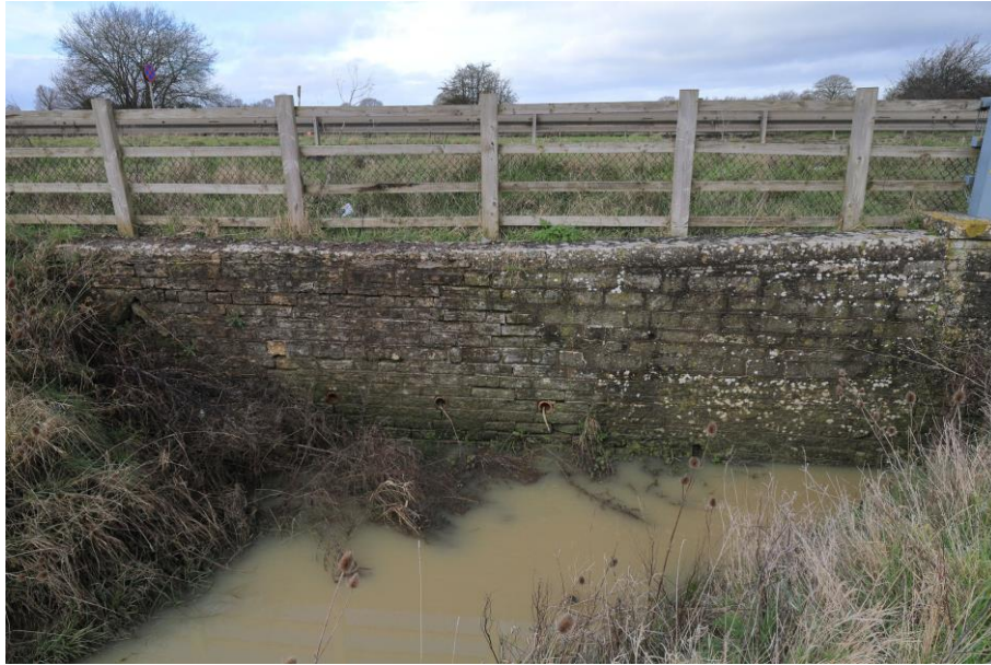
Figure 17: Stone block mortared wall showing significant signs of instability (A303, SGM 1268, January 2021).
