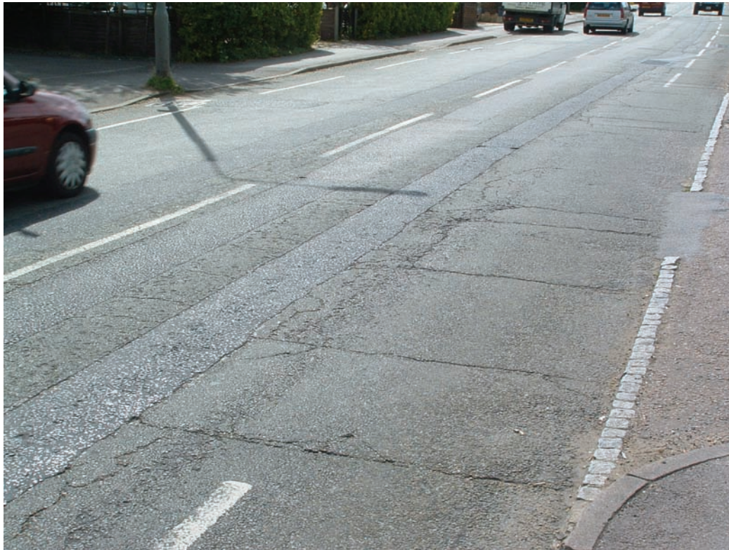
Figure 3 Cracking in the zone of influence adjacent to one of the longitudinal reinstatements shown in Figure 1
