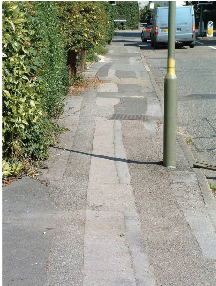
Figure 11 A footway with multiple reinstatements
