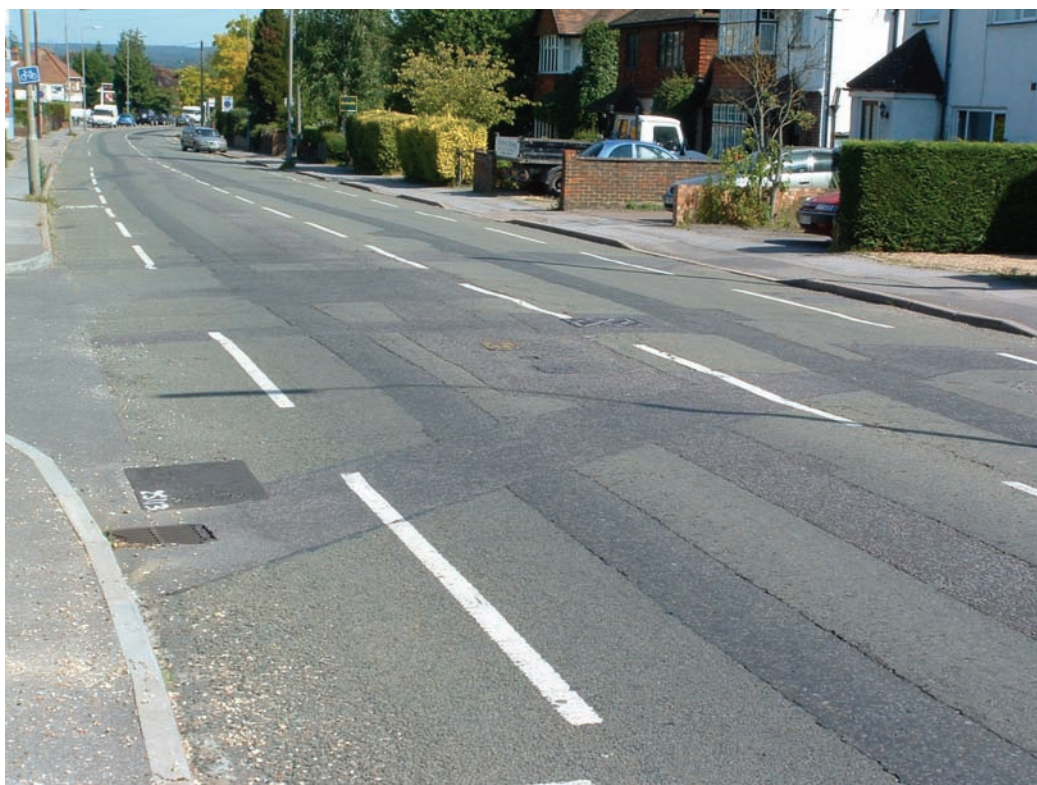
Figure 2 The carriageway shown in Figure 1 with intersecting longitudinal and transverse reinstatements
