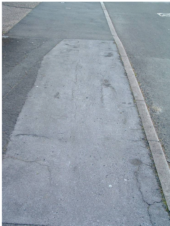
Figure 12 Reflection cracking at an old reinstatement in a footway after surface treatment
