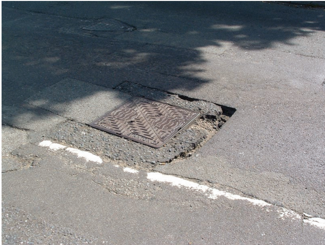
Figure 7 Potholing in a carriageway adjacent to ironwork
