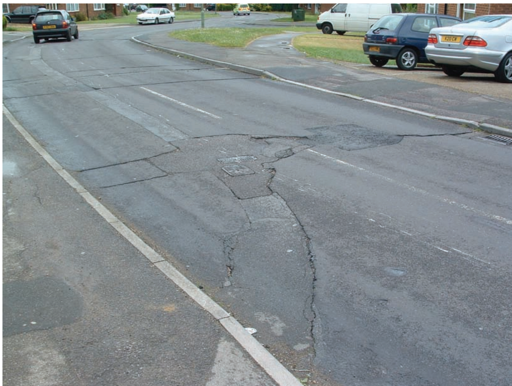
Figure 6 Surface deterioration at a reinstatement near ironwork in a carriageway with a concrete pavement and an asphalt overlay
