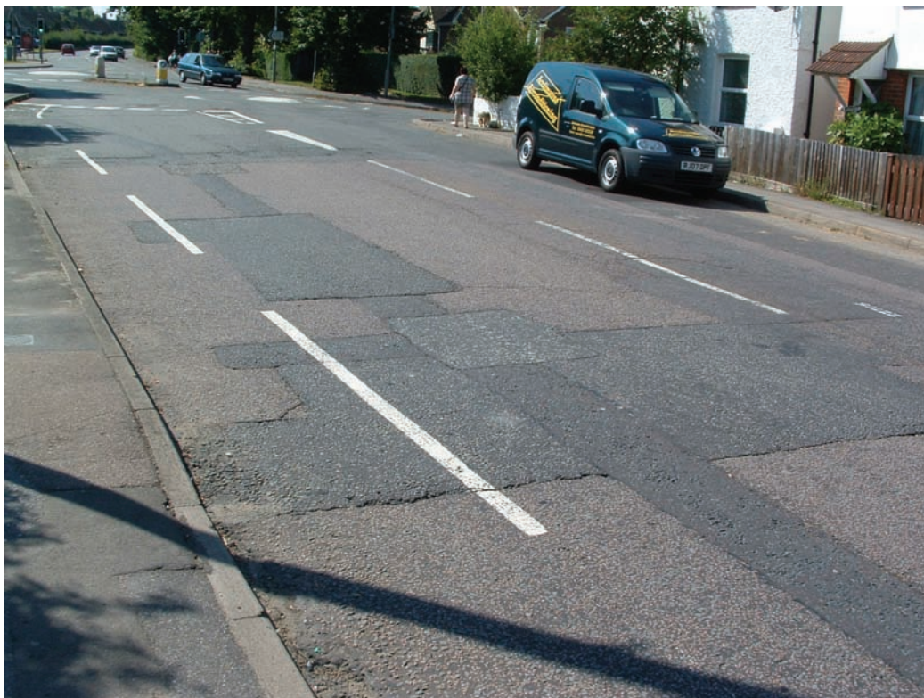
Figure 4 A reinstated carriageway with multiple repair patches
