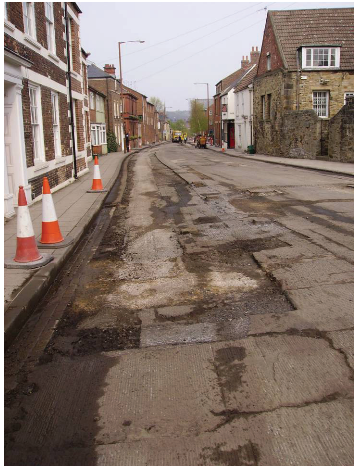
Figure 10 Repairs being made to the reinstatement and the binder and surface courses in the carriageway shown in Figure 9 (viewed from the opposite end of the street)
