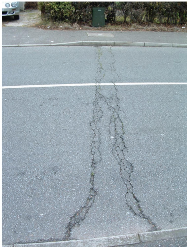
Figure 8 Reflection cracking at an old reinstatement in a carriageway after resurfacing
