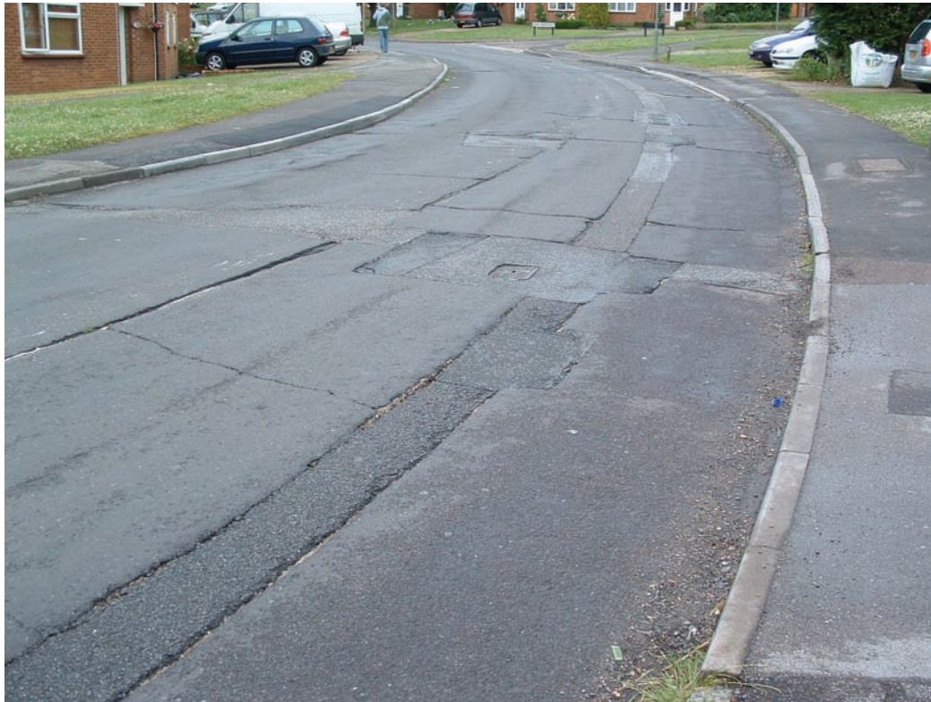
Figure 5 Surface deterioration at a reinstatement in a carriageway with a concrete pavement and an asphalt overlay
