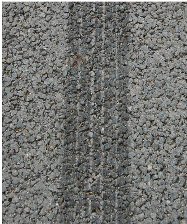
Figure 5: The Stone Mastic Asphalt surface, together with mark from car tyre
