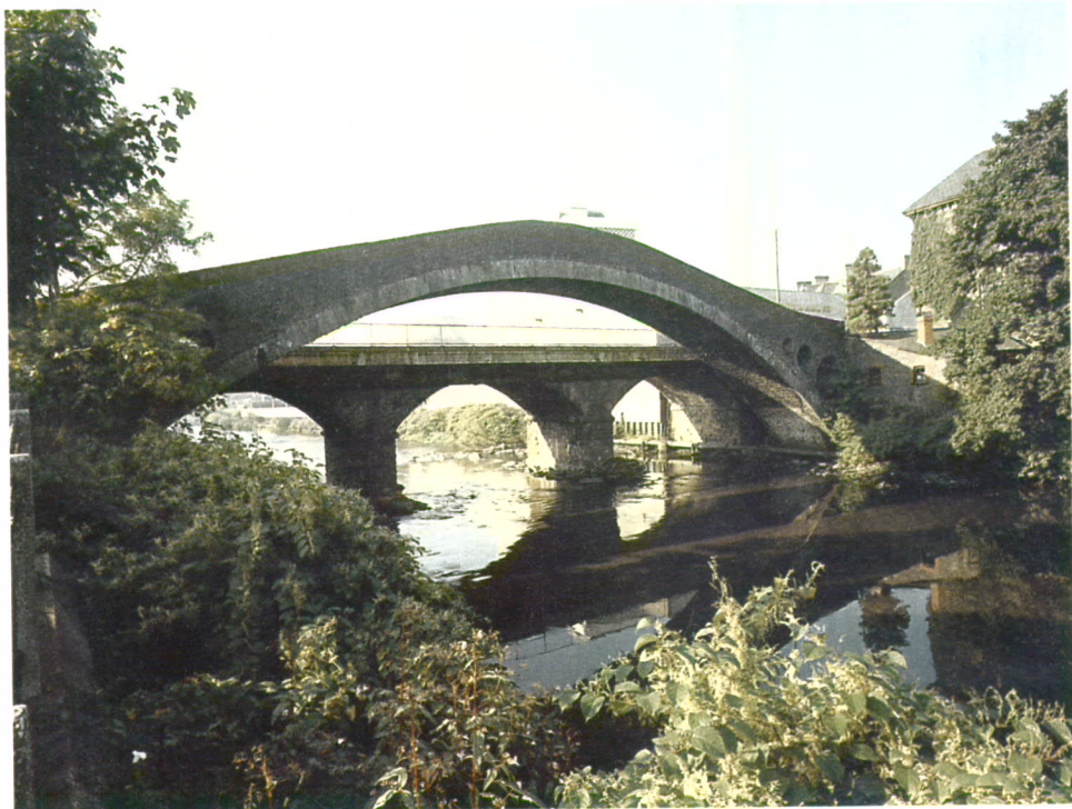
Fig.2 Pontypridd Bridge, with cylindrical voids in the fill at the haunches
