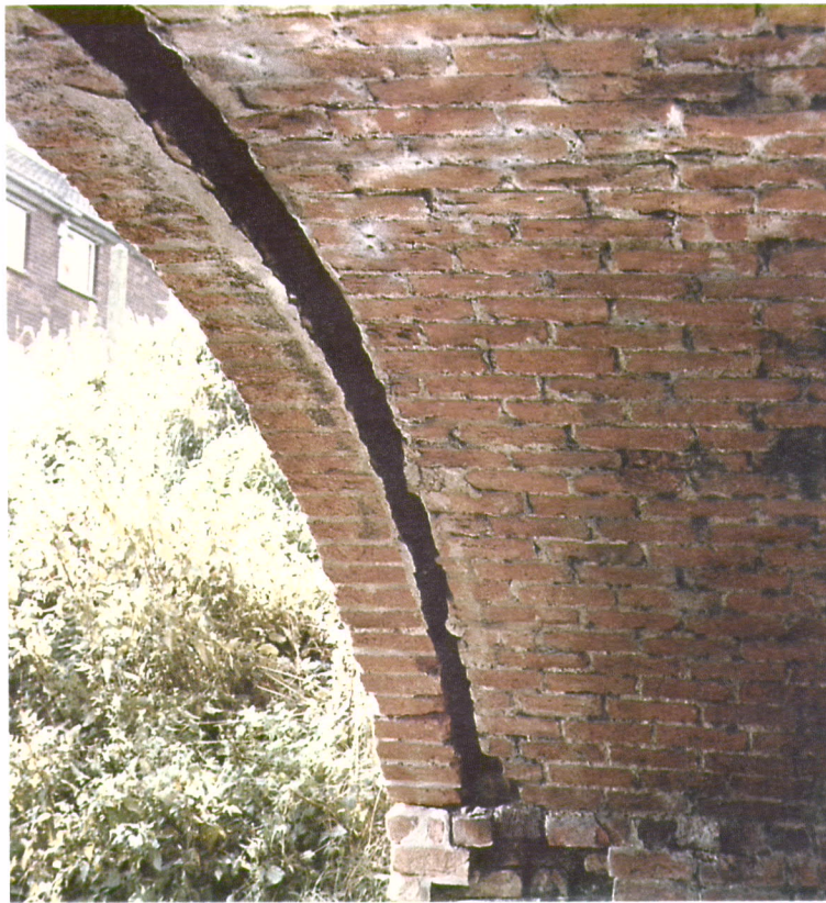
Fig.7 Severe longitudinal crack in arch ring due to outward movement of spandrel wall
