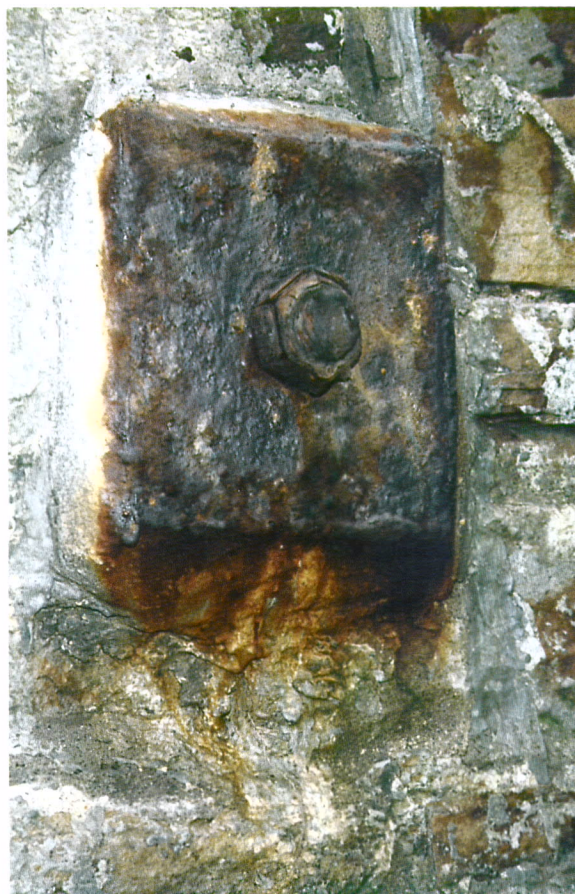
Fig.19 Rusting pattress plate
