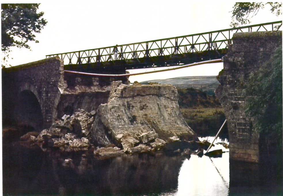
Fig.5 Collapse of arch bridge pier due to river in flood
