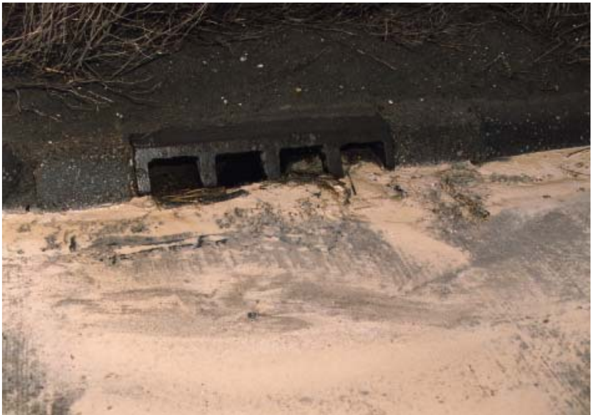
Photograph 22 Waterborne arisings running into gully outlet
