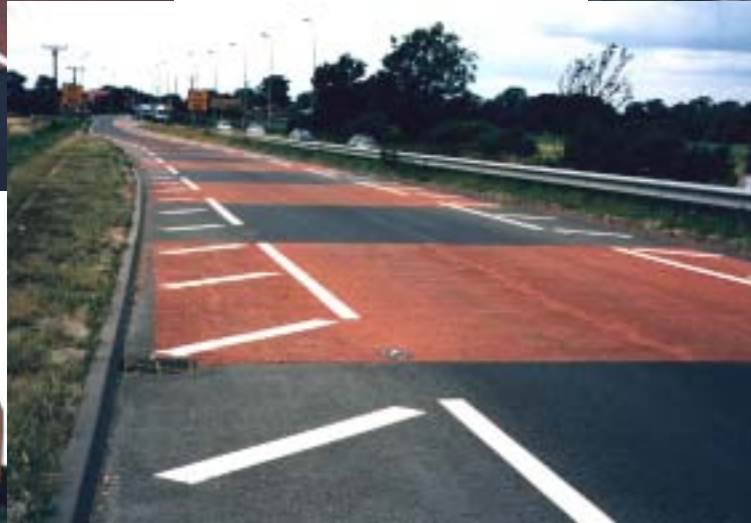
About halfway along the red patches in advance of the southeast gateway on the dual carriageway approach
