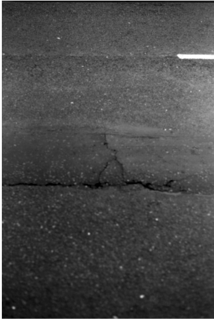
Figure 7 Crack emerging on Greenford Road
