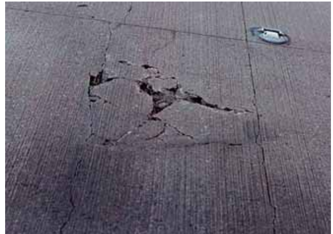
Figure 2.2 Localised failure due to punchouts
