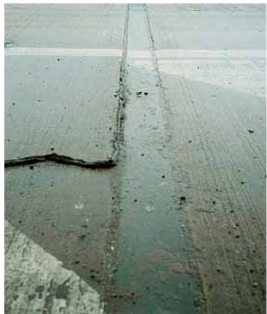
Figure 8.4 Debonding of the joint sealant at the WFB
