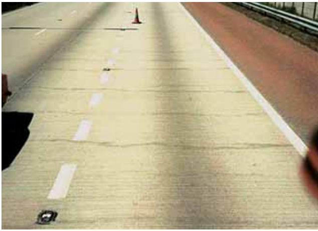
Figure 2.1 Transverse cracking in CRCP
