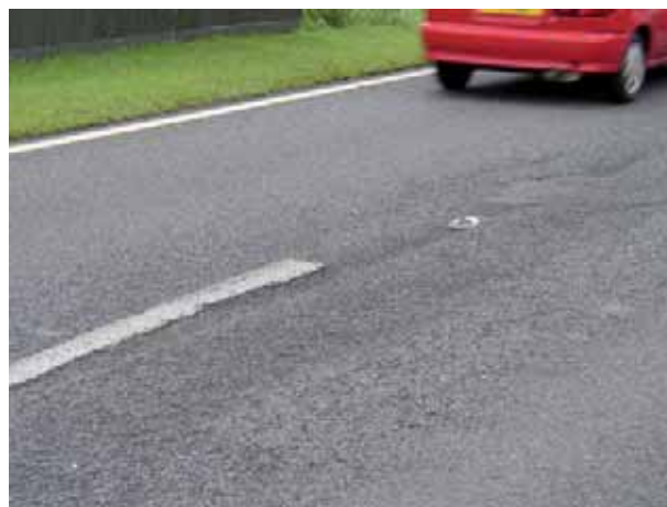
Figure L.2 Widespread particle loss on A5
