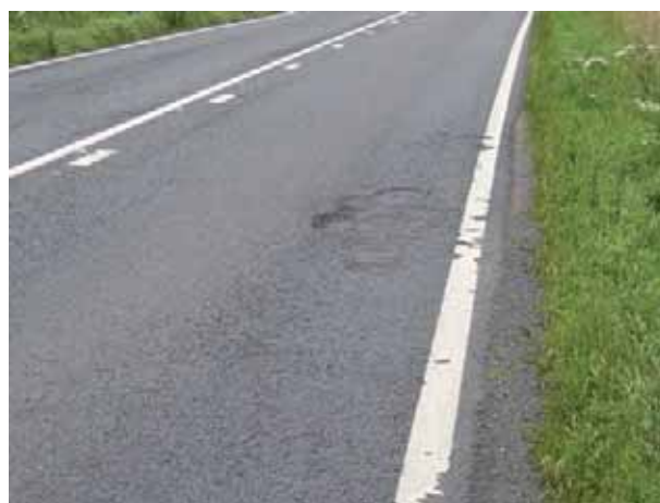
Figure L.3 Development of potholes on A5
