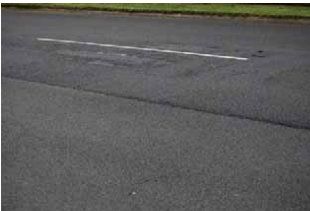
Figure 9.3 Example of site in Suspect condition
