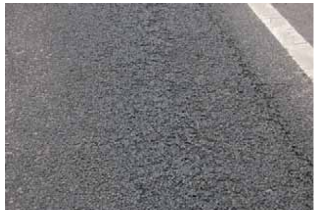
Figure 9.4 Example of site in Poor condition
